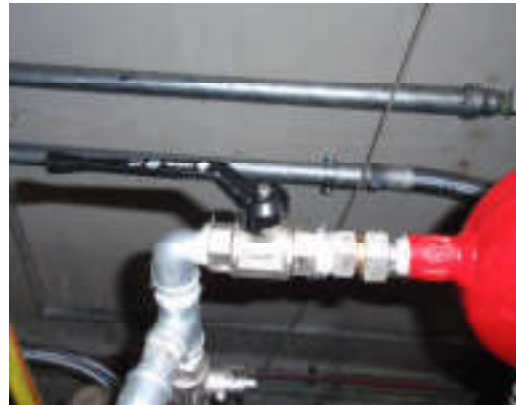
Alarm mute valve
