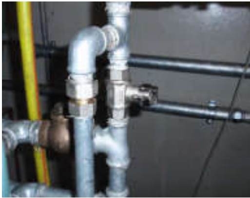
Alarm test valve "anti-tampering"
